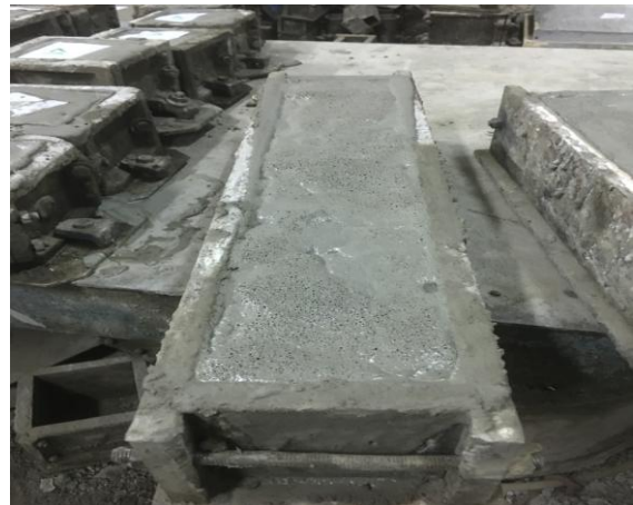
Fig 1: Formed bubbles on the concrete surface after pouring the concrete
