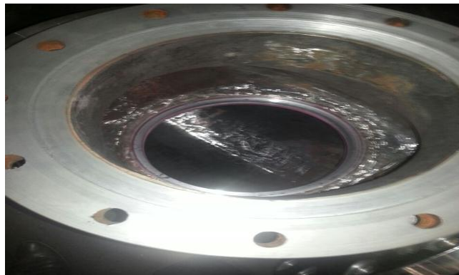
Fig 1: Damage at the seal seat of a globe valve due to wear
