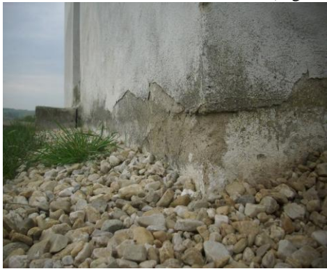
Fig 3. – Damages on external surface (Author: Ladislav Tazky)
