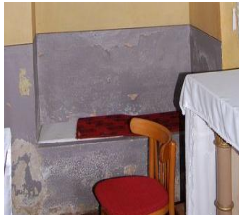
Fig 6. – Damages on internal surface of the church (Author: Ladislav Tazky)
