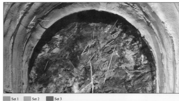
Fig. 4. A face of tunnel excavation at Polimilos Part of Egnatia Highway at Northern Greece
