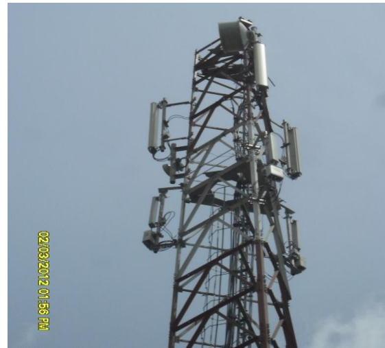
Fig 2: Base station used for the experiment: ASA 001
