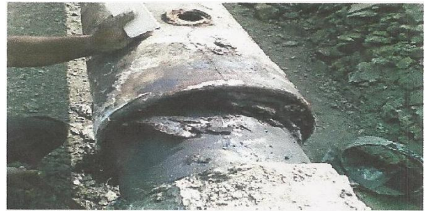
Fig. 4 Condition of partial shorted casing after excavation Remedial Measure to remove the shorting:
