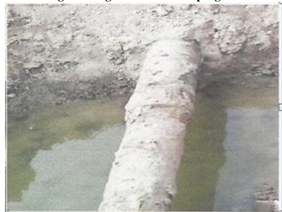
Fig. 6 Condition of casing of old pipeline
