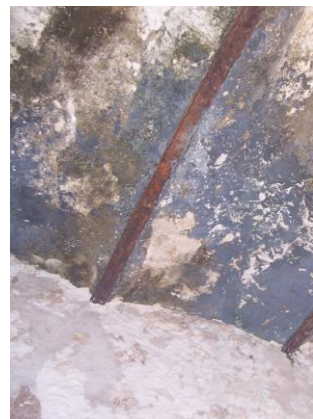
Fig 3: Condensation, dampness and mould growth on the slab of the Old Boma
