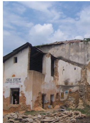
Fig 1: Incurably deteriorated historic building falling apart inside and out in Bagamoyo, Tanzania
