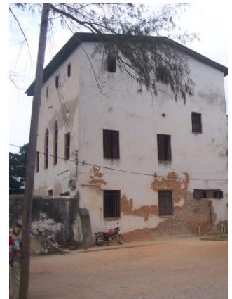
Fig 2: Lime plaster falling off the external wall of the Old Fort in Bagamoyo, Tanzania
