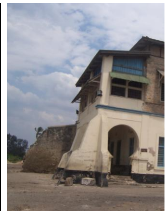
Fig 4: Use of cement sand blocks not similar to the original limestone on German Customs House in Bagamoyo, Tanzania
