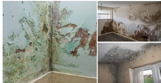
Fig.1. Dampness in masonry
