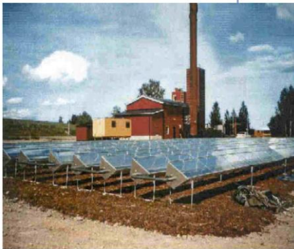
Fig 6: Solar collectors array
