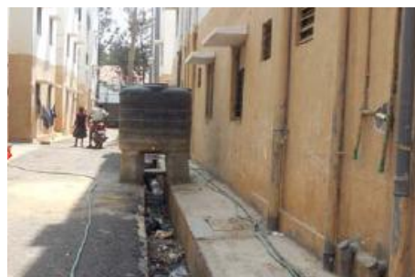
Fig. 6 Open drains are filled with Solid Waste
