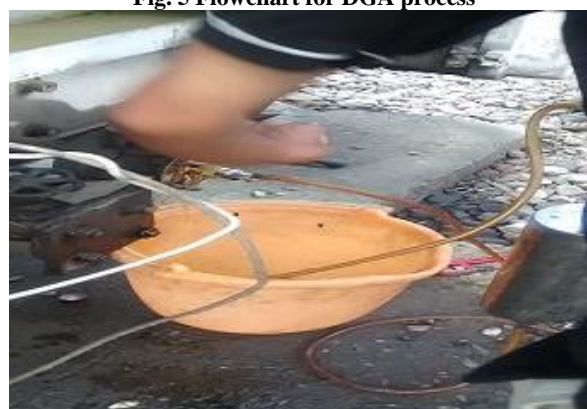
Fig. 6 Sampling at Anoo substation, Hamirpur, HP, India
