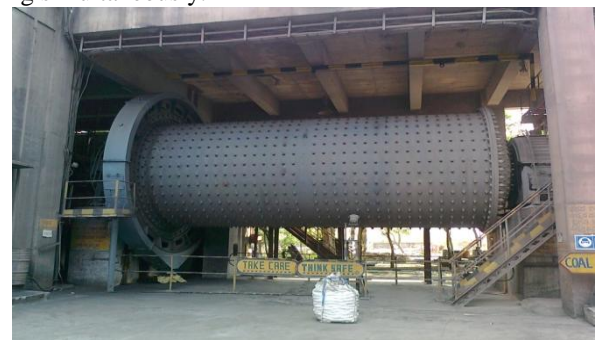
Horizontal Coal mill
