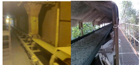
Belt conveyor transferring the material to raw mill
