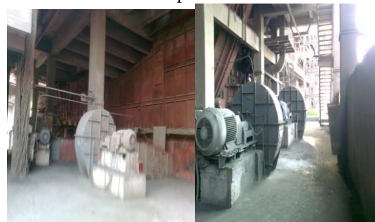
Cooler fans for cooling the material from kiln
