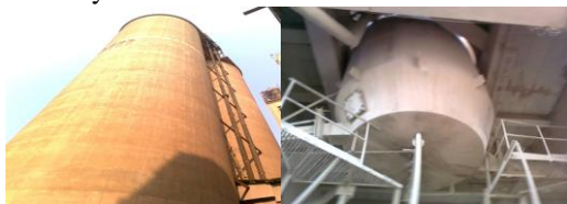
Raw meal silo weigh bin
