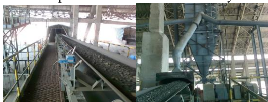
From clincker silo to cement mill trough belt conveyors
