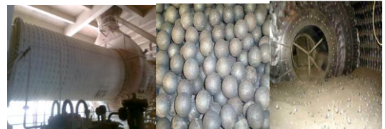
Raw mill grinding media
